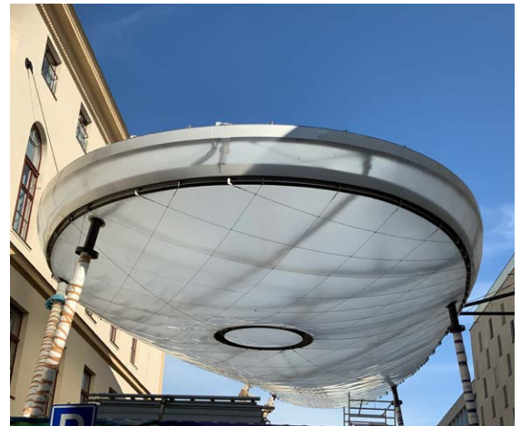
Six filigree columns and tie rods connected to the nearby buildings support the art installation »The Cloud« in the courtyard of the arts-and-crafts museum in Brno.
