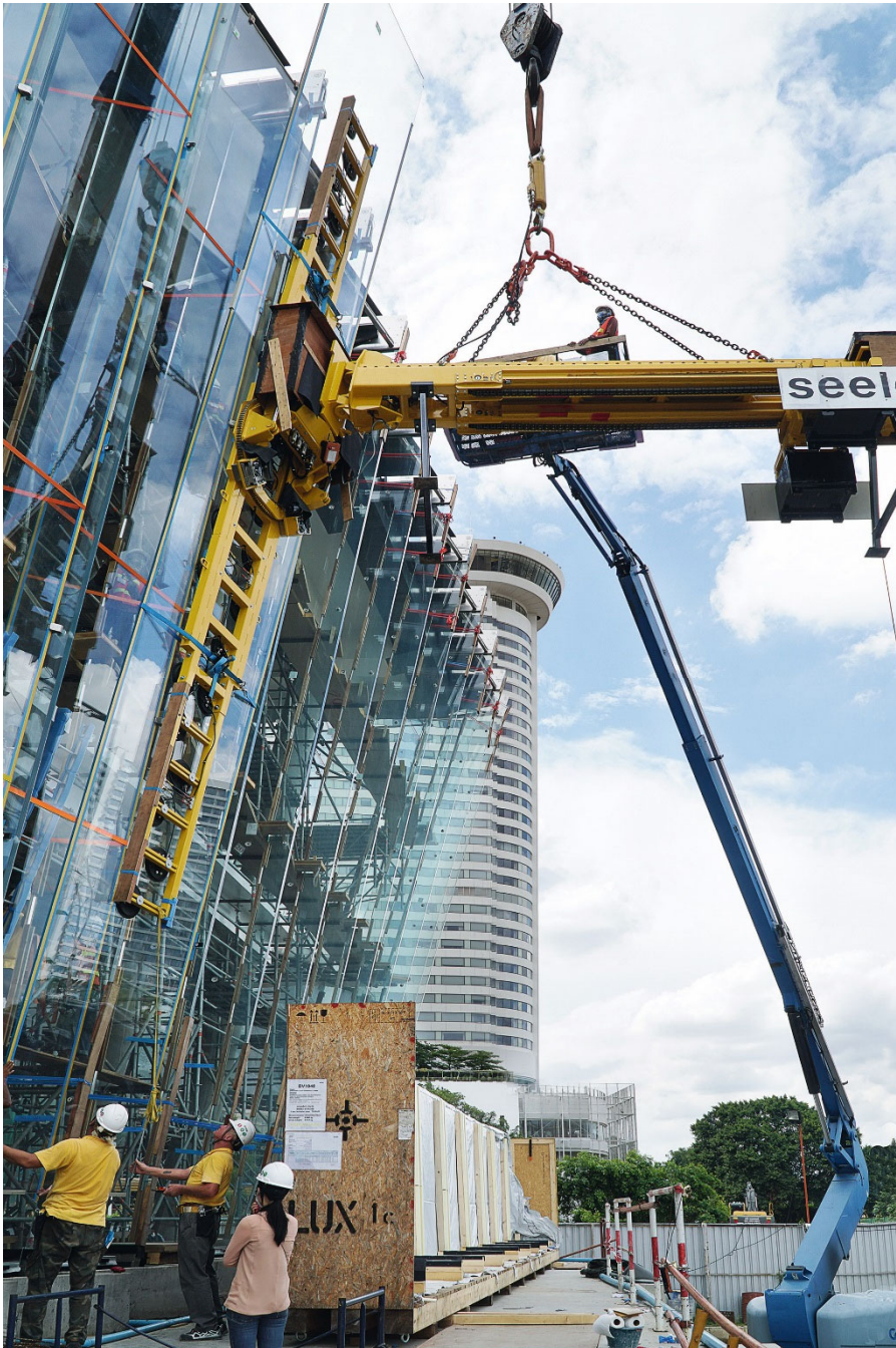
Assembly of the glass panes: The specially manufactured suction unit turns the glass into the required geometry for installation into the façade. © seele
